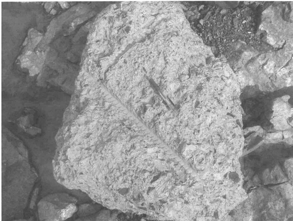
Photo 11 – Apron RCC Showing Separation at the Steel Level
