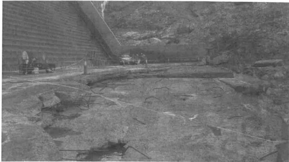
Figure 8 – Damage to Dissipator Slab from 2013 Flood
