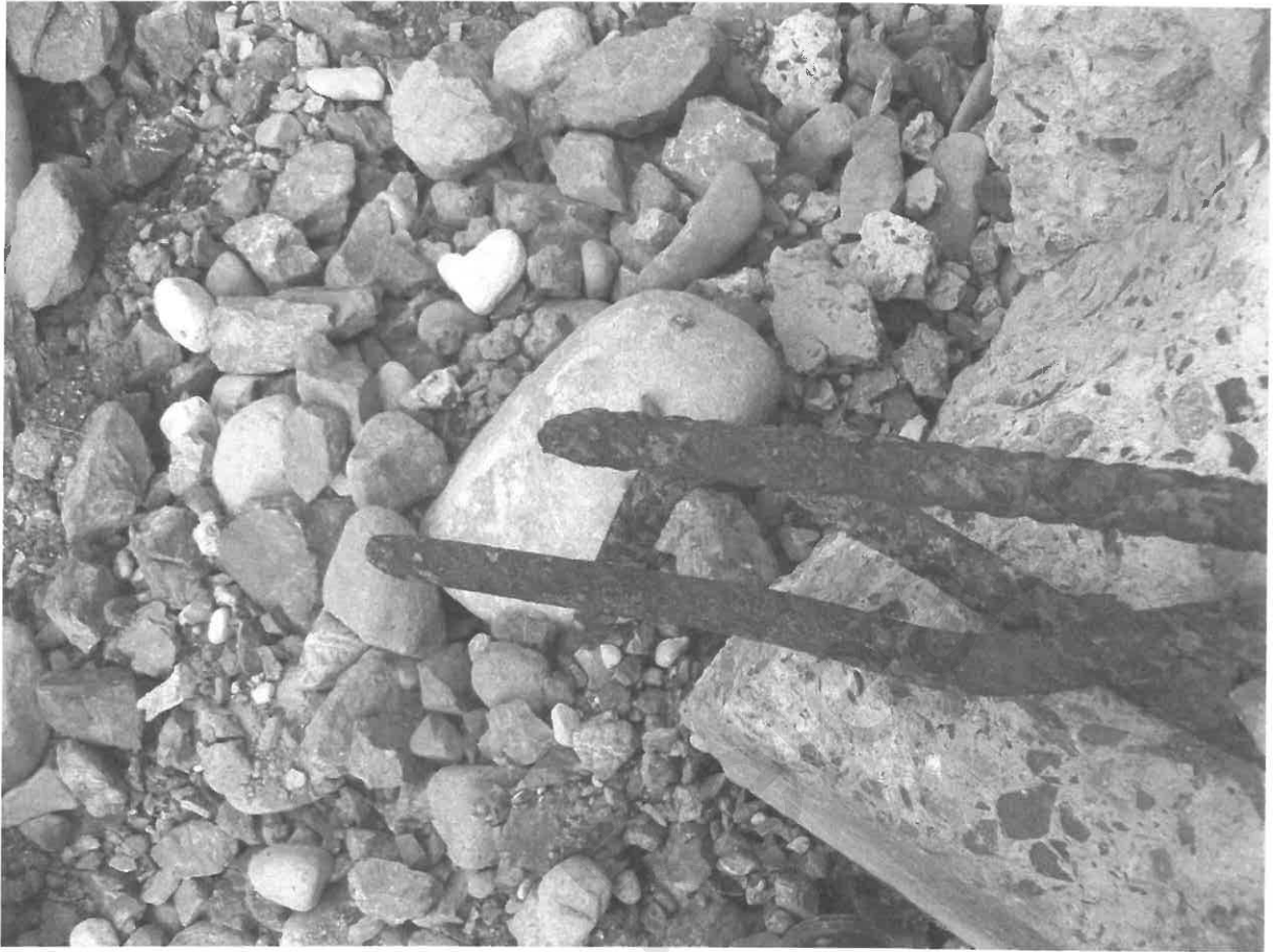
Photo 8 – Necking of Reinforcement Bars Indicating Tensile Overload
