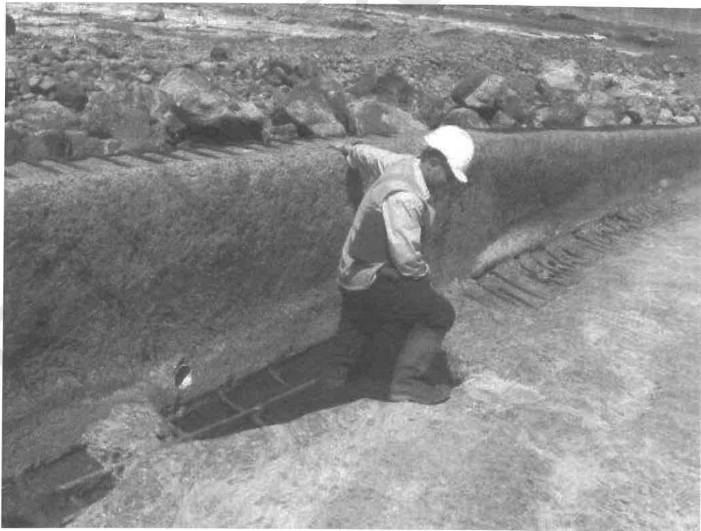
Figure 3 – Abrasion through Dissipator Apron
