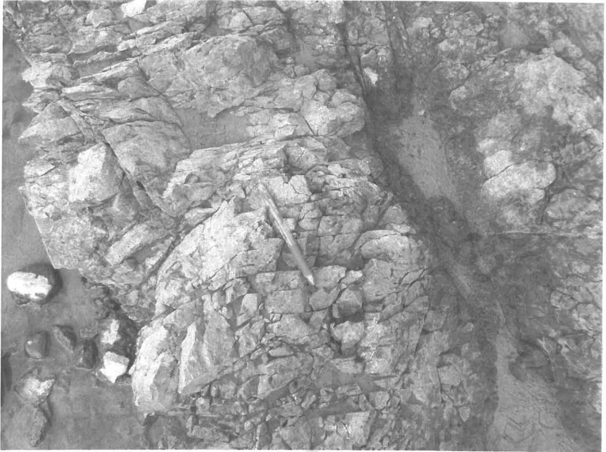
Photo 10 – Closely Fractured Rock Less Resistant to Scour
