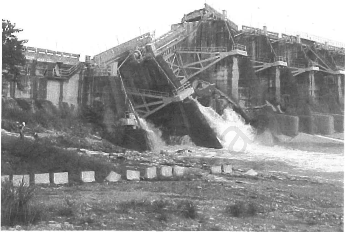
Figure 11 – Earthquake Damage to Shih-Kung Dam Taiwan
