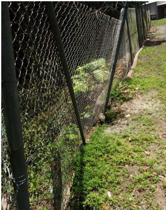
South Mossman river bank collapsing beneath boundary fence, adjacent the oxidation ditch and lagoon.
