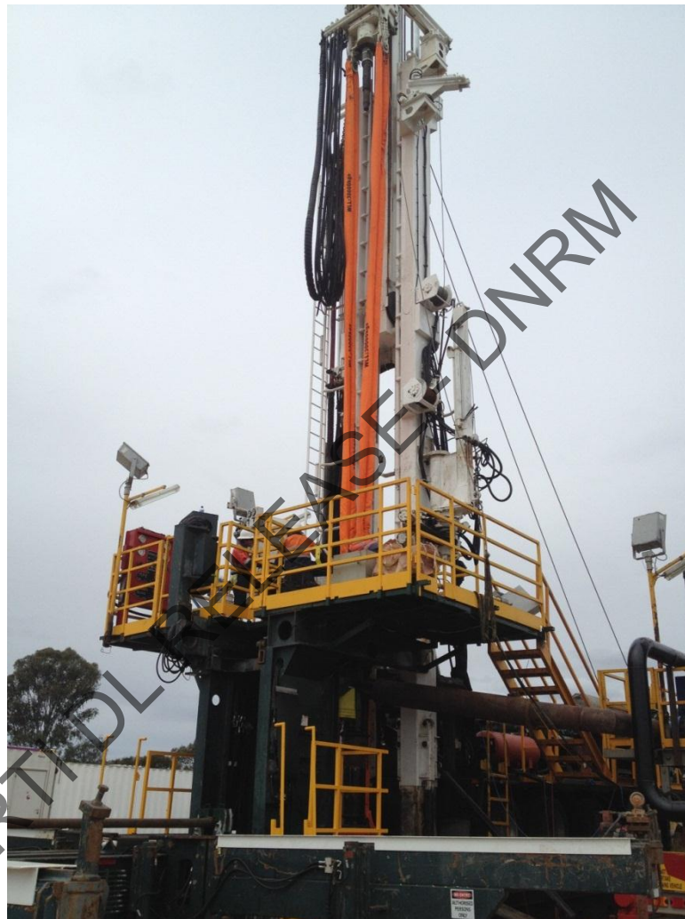
Photograph 3. General view of Shramm Drill Rig TXD 01, in preparation for Static Load Test on Mast Structure showing Pull Up Slings used during this activity.
