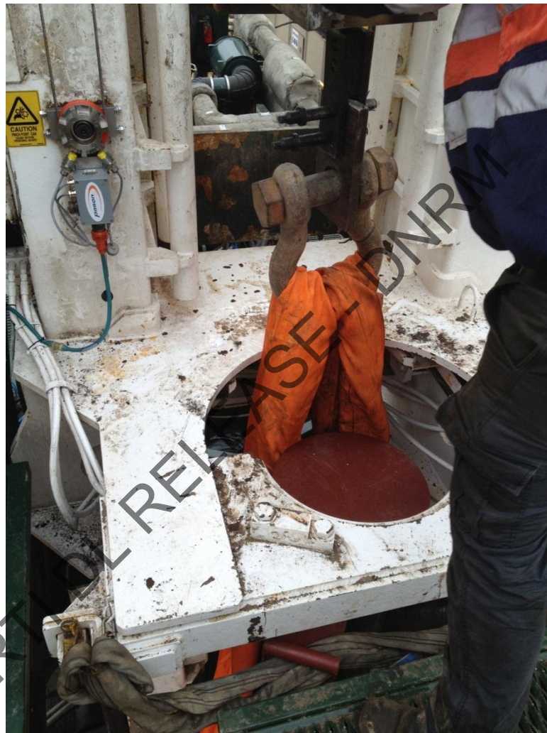
Photograph 6. General view of Shramm Drill Rig TXD 01, in preparation for Static Load Test on Mast Structure showing Hold Back Slings, Shackle, Transmission Link used during this activity.
