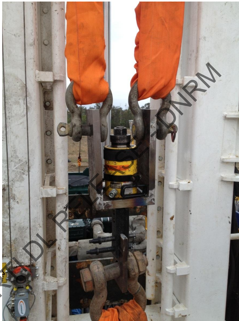
Photograph 4. General view of Shramm Drill Rig TXD 01, in preparation for Static Load Test on Mast Structure showing Pull Up and Hold Back Slings, Shackles, Load Frame, Transmission Link and Load Cell used during this activity.
