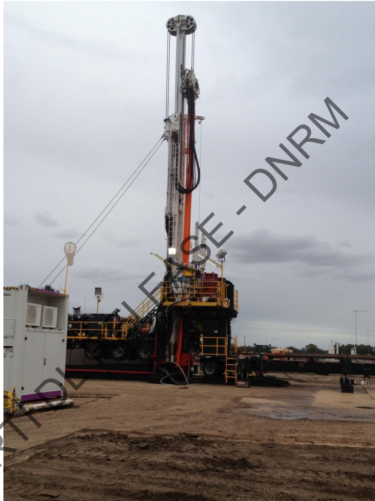
Photograph 2. General view of Shramm Drill Rig TXD 01, in preparation for Static Load Test on Mast Structure showing Pull Up Slings used during this activity.
