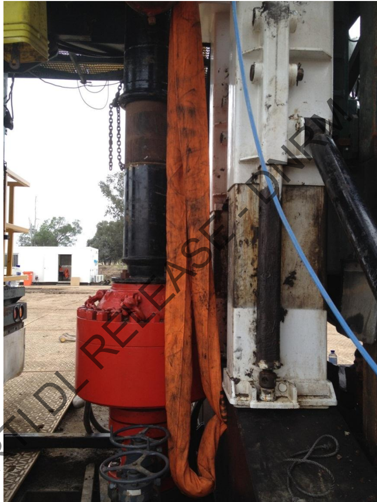
Photograph 7. General view of Shramm Drill Rig TXD 01, in preparation for Static Load Test on Mast Structure showing Hold Back Slings at Lower Securing Point (Sub Base) during this activity.
