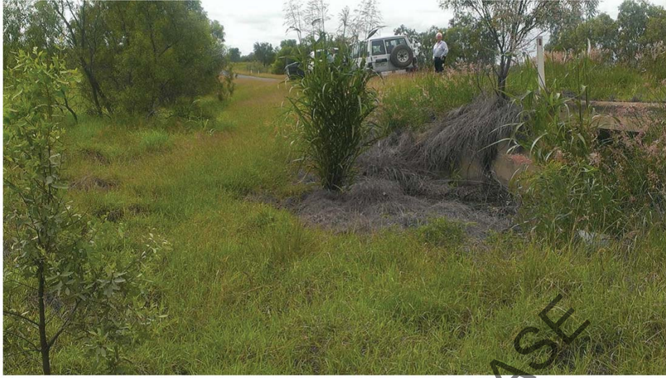
Perched culvert on lillyvale road
