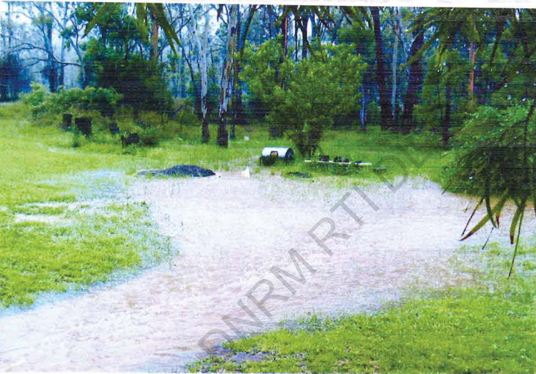
Photo 5 showing general rain run of from culvert, current temporary track top left of photo
