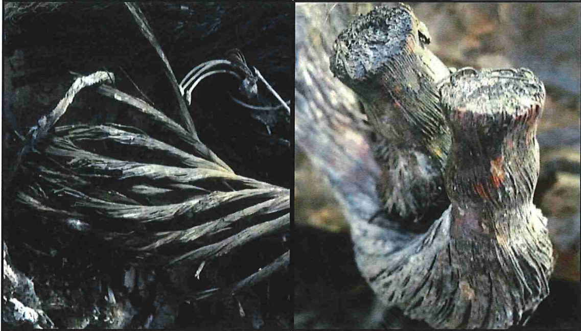
Figure 44 – Copper cable showing (a) pulling and stretching (b) separation from battery terminal.
